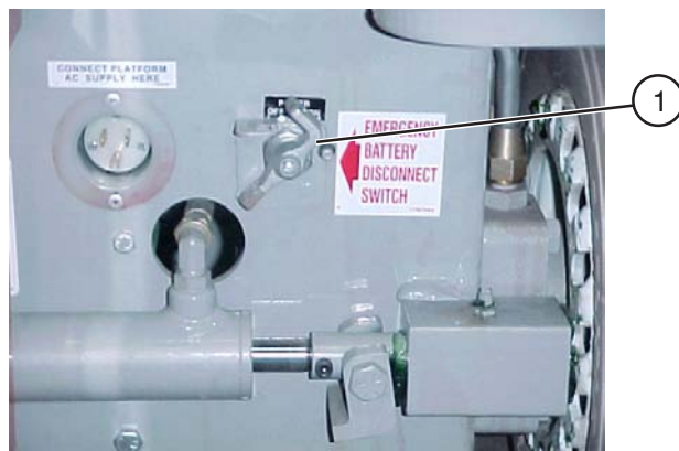
Figure 2-2. Emergency Battery Disconnect Switch
